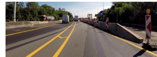
Use of a temporary concrete safety barrier combined with type la.2 panel along the crossing of the central reserve
